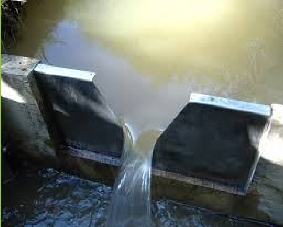
'V' Notch for Flow Measurement
